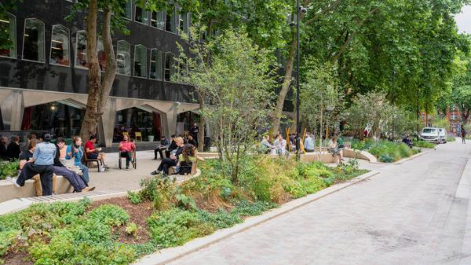
Redesign of street removing general traffic and repurposing space for active travel, seating and planting which incorporates existing mature trees, Alfred Place, London
