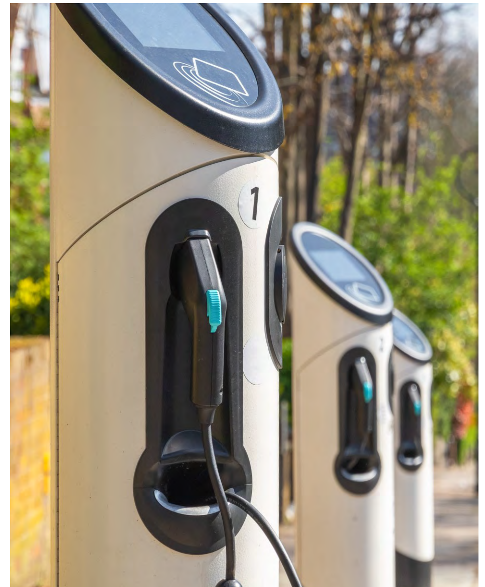
Figure 3 EV Charging Point
